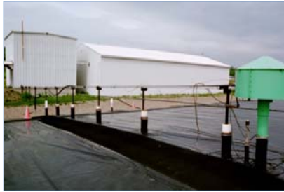
Trench 14 leachate pump line
