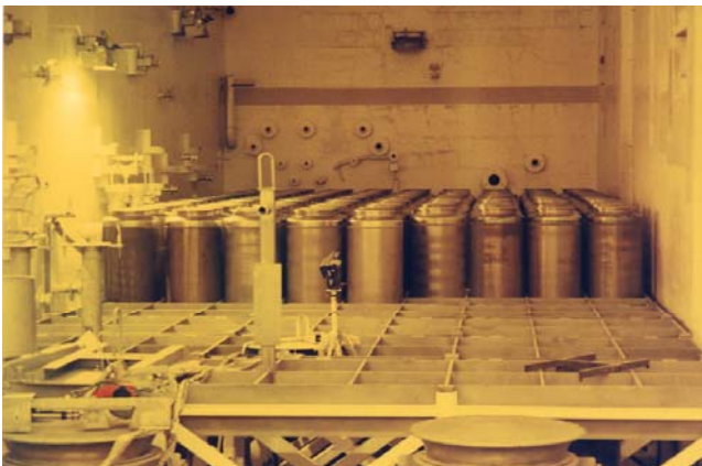
275 HLW canisters are safely stored inside the Main Plant Process Building
