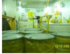
Workers load waste from the cleanup of the Process Mechanical Cell Crane Room into a Standard Waste Box
