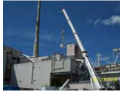
A Standard Waste Box is removed from the Process Mechanical Crane Room Extension
