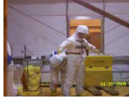
Operators processed low-level waste boxes in containment structure to prepare for actual CH-TRU waste processing in the newly-modified facility
