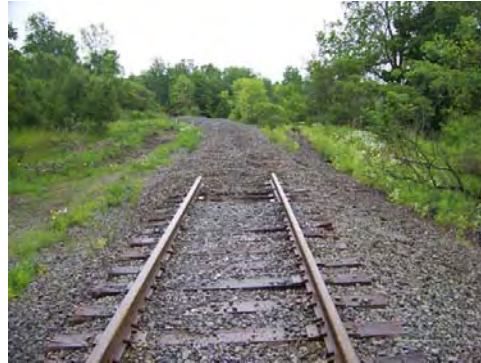
Rails and ties have already been removed from the repair area at the landslide location
