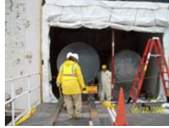
Two vessels were removed from the Hot Acid Cell, immediately packaged, and disposed within two weeks
