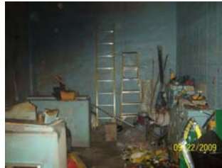
Debris cleanup and removal of tank pieces from the Acid Recovery Cell are in progress.
