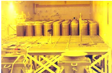
275 HLW Canisters in Safe Storage in Main Plant Process Building
