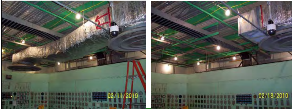
Main Plant Control Room, before and after control panel and ventilation removal
