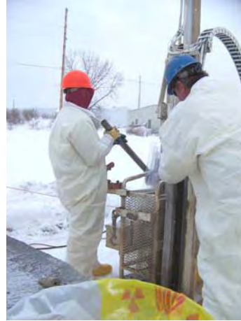
Specialized drillers remove 4' long sections of soil, to determine depth of till
