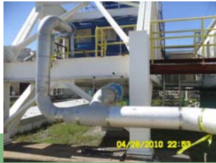
New ventilation lines installed in Tank Farm to prepare for connection to T&VDS
