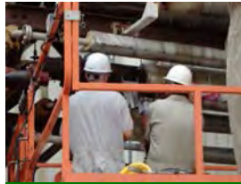
Utilities Isolated and Air-Gapped
