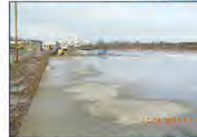
Five separate concrete placements and more than 300 concrete delivery trucks involved in completing the HLW Storage Pad and Approach Apron.
