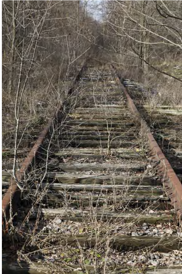
Rails need to be removed from the trail between Jewett Holmwood Road and Bank Street in Orchard Park. (Derek Gee/Buffalo News)
