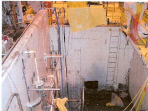
FRS Pump Pit
