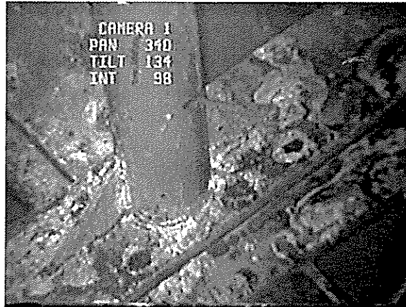
Circular tank about 70' in diameter, 27' high
