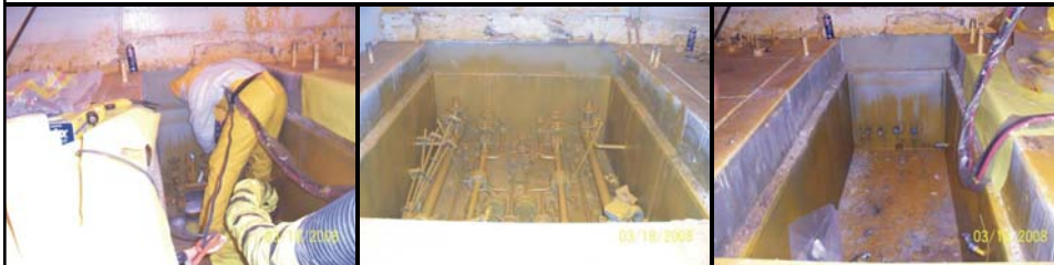
Decontamination of a pump niche in the Upper Warm Aisle in the Main Plant Process Building
