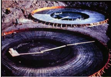
Underground waste tanks
