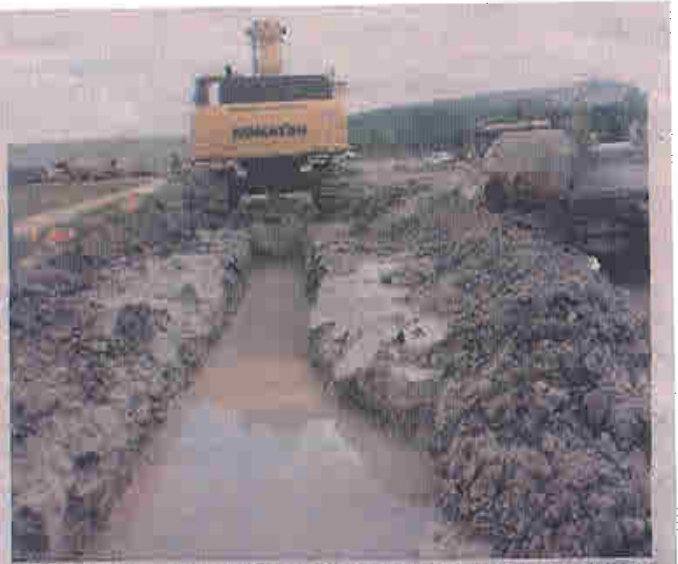
CLAY WALLS — Excavation of the slurry wall in progress at West Valley Demonstration Project. WVDP file photo.
