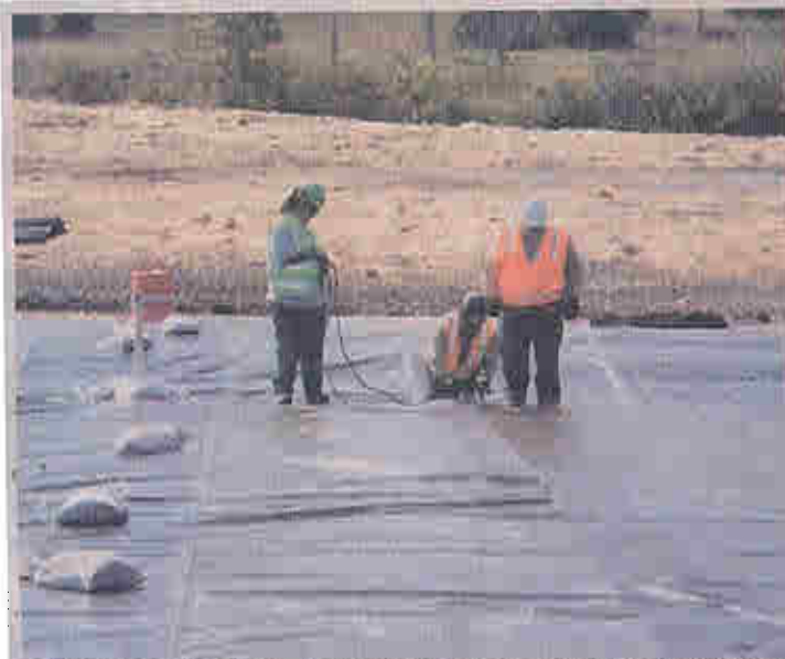
FINISHING TOUCHES — A West Valley Demonstration Project work crew welds the geomembrane panel together. WVDP file photo.
