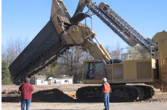
One Pass Trencher – A trencher capable of excavating and backfilling the trench in a continuous motion will be used to construct the PTW.
