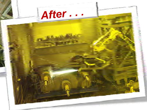
Electrodes removed, melter removed from Vitrification Cell, packaged and placed on hardstand – ready for shipment
