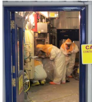
Electrical Isolations – 01-14 Building
