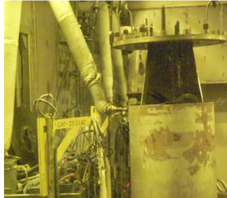
Decontamination of the Submerged Bed Scrubber fuel basket in the vitrification cell
