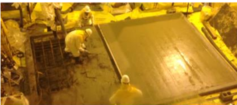
Installed Equipment Decontamination Room (EDR) Soaking Pit Cover
