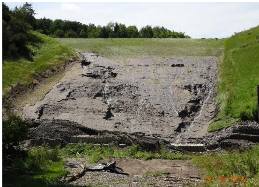
Lake 1 Spillway After the Storm
