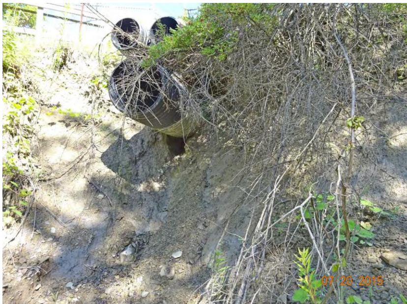
Additional Erosion of S-09 Discharge Pipes Caused by the Storm
