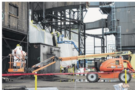
A crew is doing asbestos work at the Portsmouth Gaseous Diffusion Plant in Piketon.
