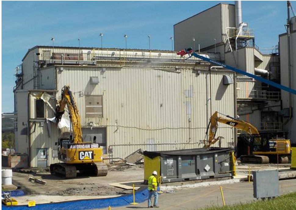
Demolition of the Vitrification Facility begins with the "first bite" on Sept. 11.
