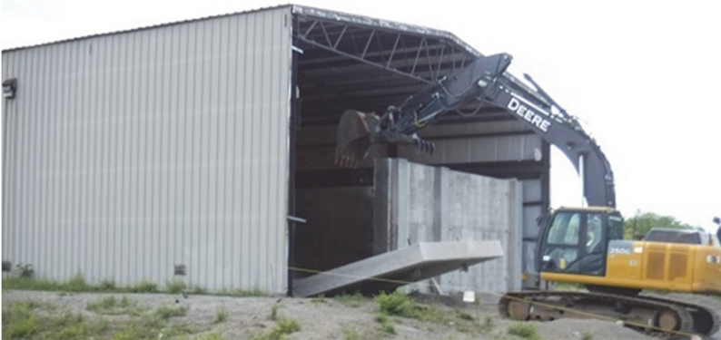
An operator at the West Valley Demonstration Project uses an excavator to remove a large concrete shield wall to create an entrance to accommodate a large fork truck for transporting empty waste containers in and out of the building.
