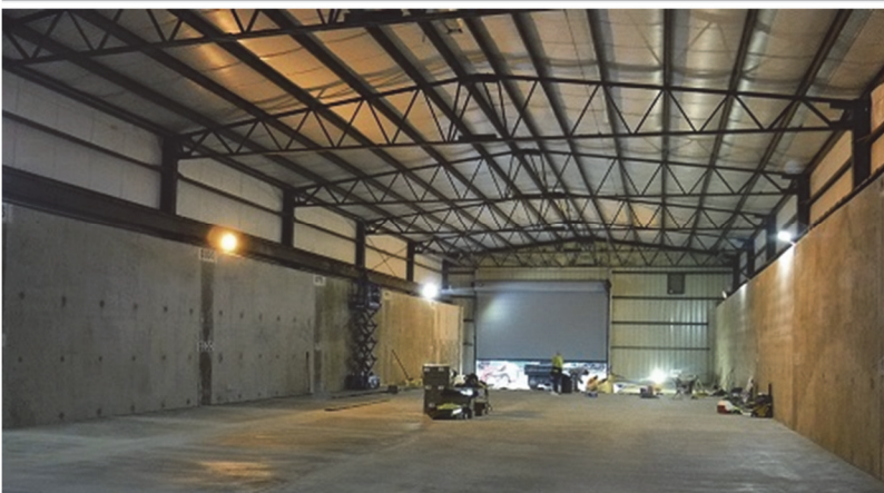
Crews renovate a former storage facility for waste disposal operations at the West Valley Demonstration Project. A new roll-up door is in the background.
