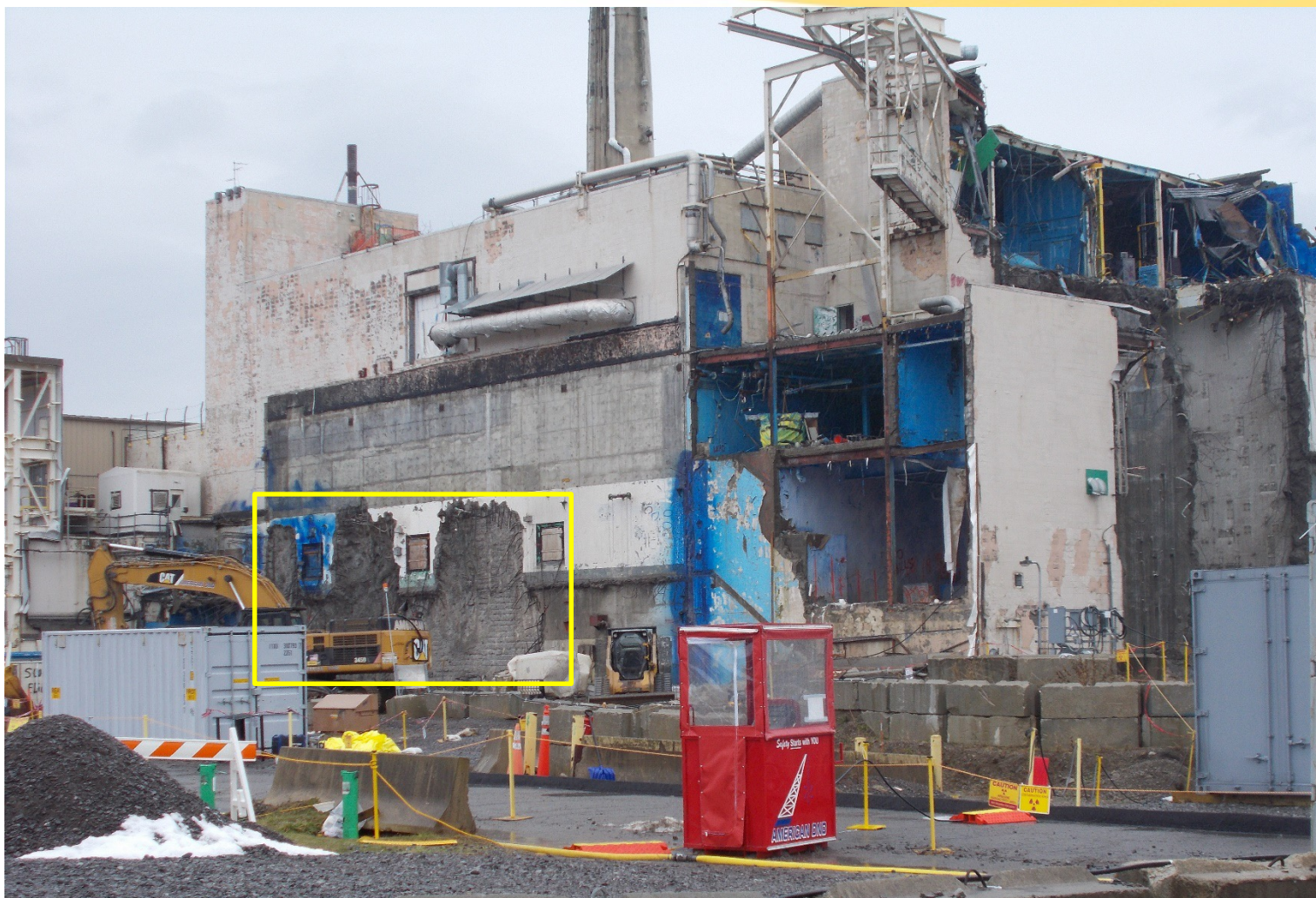
Deconstruction of the Chemical Process Cell west wall by removing the first three (3) feet of wall of the 5-foot-thick wall
