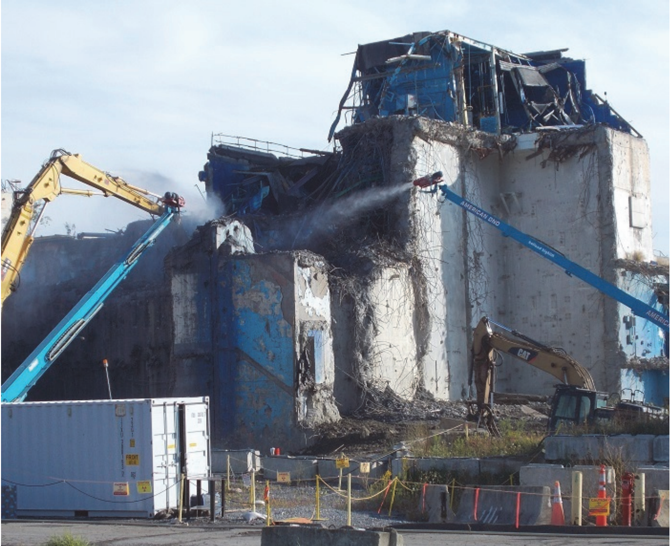
EM team members continue to demolish the Main Plant Process Building at the West Valley Demonstration Project as they begin removing hot cells within the facility's analytical laboratory. Those cells were used during past fuel reprocessing and vitrification operations. A hot cell is a highly shielded room where activities involving high radiation levels can be safely performed.
