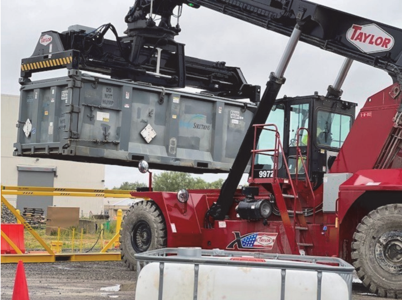
An EM worker uses a long-reach fork truck to transport full waste boxes from the Main Plant Process Building demolition area at the West Valley Demonstration Project to a rail line where they are shipped offsite for disposal.
