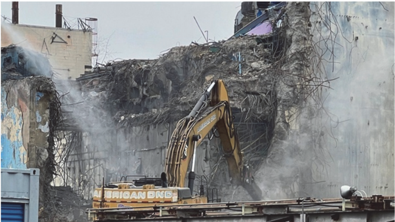
Demolition equipment using a new automated quick coupler deconstructs the wall of a cell within the Main Plant Process Building at the West Valley Demonstration Project.
