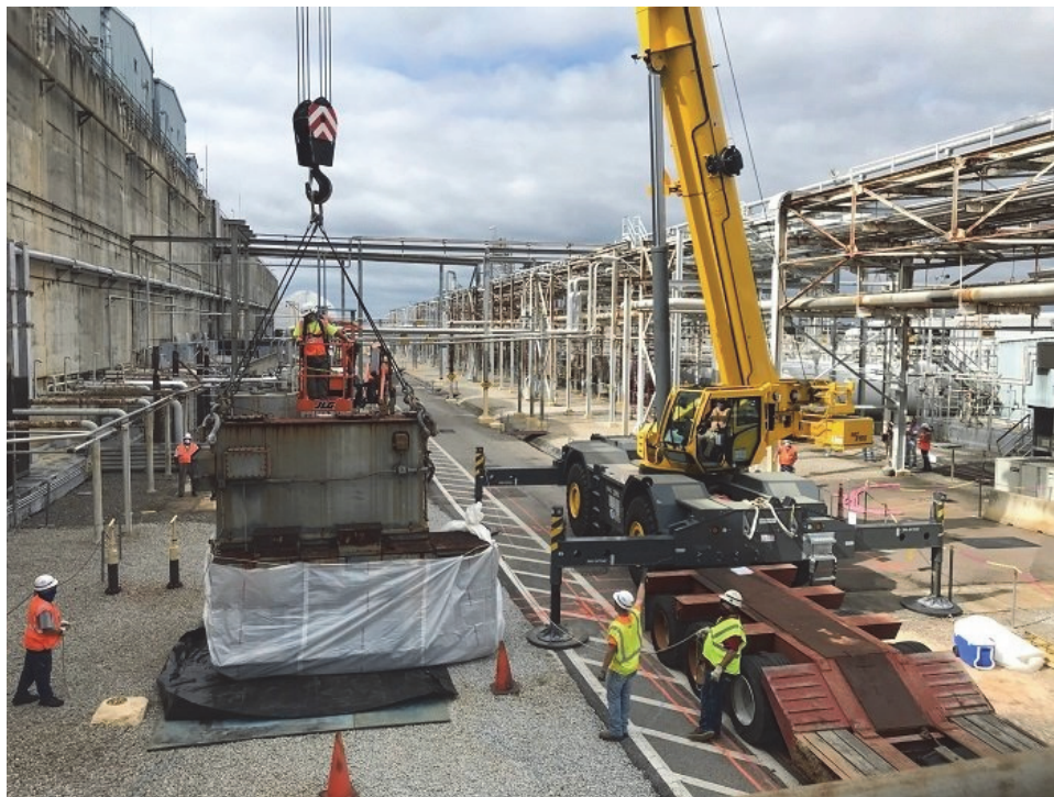
Crews at H Canyon at the Savannah River Site remove an old transformer to make room for new equipment needed for an electrolytic dissolver.
