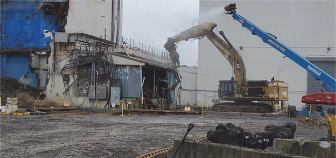
EM crews demolish the former Waste Reduction and Packaging Area at the West Valley Demonstration Project.
