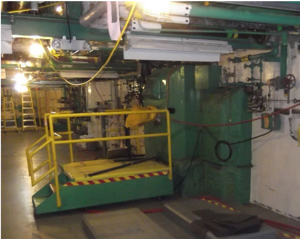
A view of the “Green Giant” inside a chemical processing cell within the Main Plant Process Building at the West Valley Demonstration Project .
