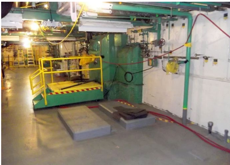
An old photo of the "Green Giant" inside a chemical processing cell within the Main Plant Process Building at the West Valley Demonstration Project .
