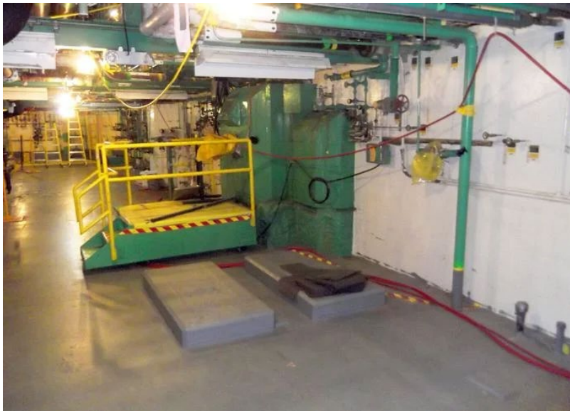
An old photo of the "Green Giant" inside a chemical processing cell within the Main Plant Process Building at the West Valley Demonstration Project .
