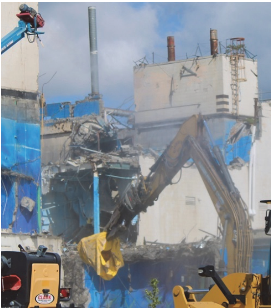
Crews use construction equipment to safely remove packaged ventilation duct sections from the Vent Wash Room as part of the demolition of the Main Plant Process Building at the West Valley Demonstration Project .
