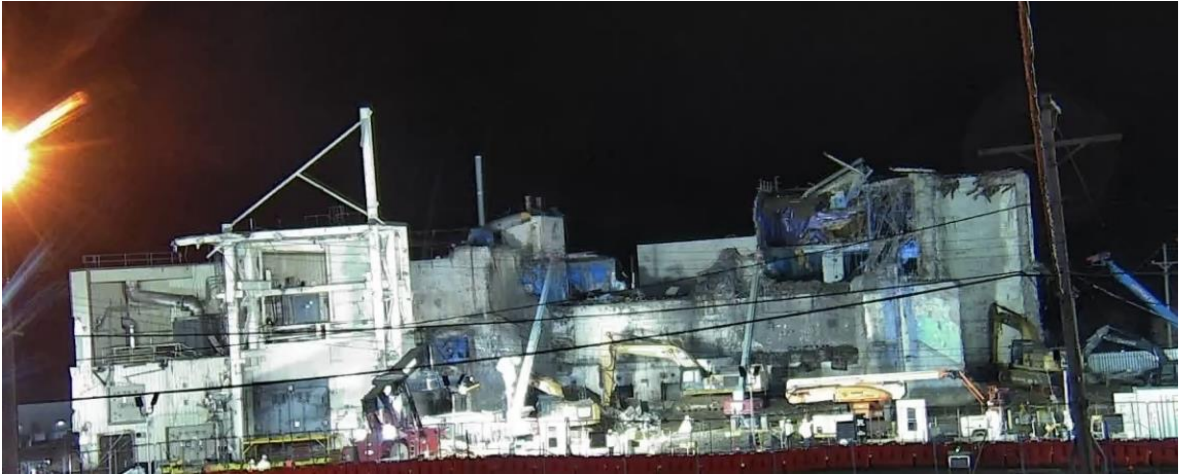
Loading Control Room and Upper Extraction Aisle debris on second shift (8:00 p.m.)
